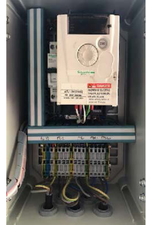
Electric box with speed variator
